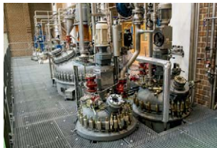
ATEX compliant installation with glass lined, pressure proof and corrosion resistant reactors (7–5,400 l) coupled to a condenser and vacuum pump.
