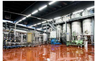
Production hall for biomass pretreatment, biocatalysis and filtration.
