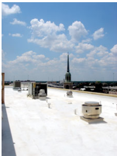
Photo of a roof system restoration after a biobased coating was installed on Baptist Medical Center's surgical wing in San Antonio
