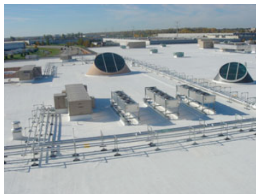
This smooth 2,600-square-foot built-up roof system on KV Pharmaceutical's building in St. Louis was restored with a biobased coating.
