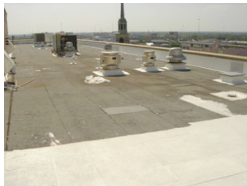
Photos courtesy of Green Products LLC, Romeoville, Ill. Photo of a roof system restoration before a biobased coating was installed on Baptist Medical Center's surgical wing in San Antonio
