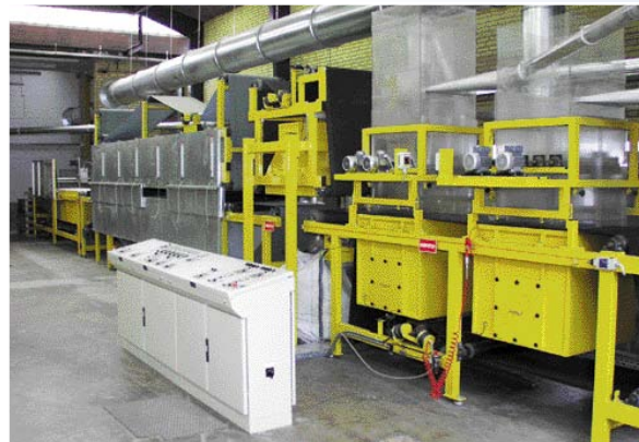
Die Mattenanlage in Saksøbing, DK The mat production facility in Saksøbing, DK
